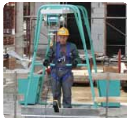
Gantry for stand hoists
