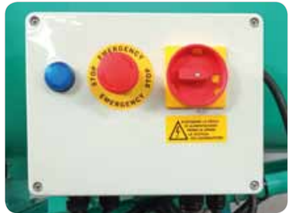
Sph Machine Control Panel
